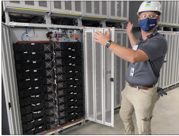
Vistra employee, Brad Masek, talks about the enormous lithium-ion battery system housed in Phase II of the Vistra Zero Moss Landing Energy Storage Facility on August 19, 2021.
